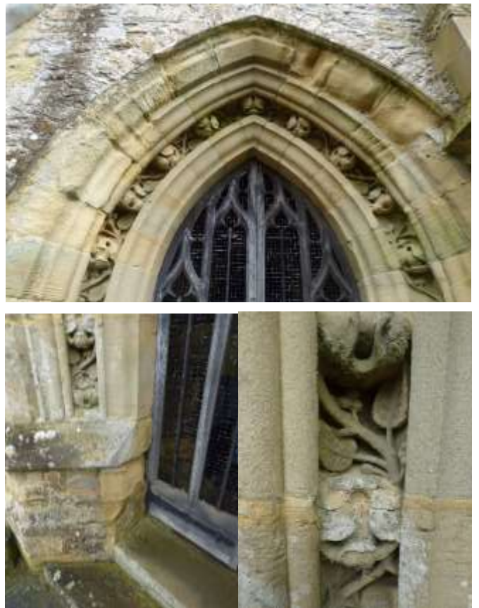
16. General views of decay to west doorway.
