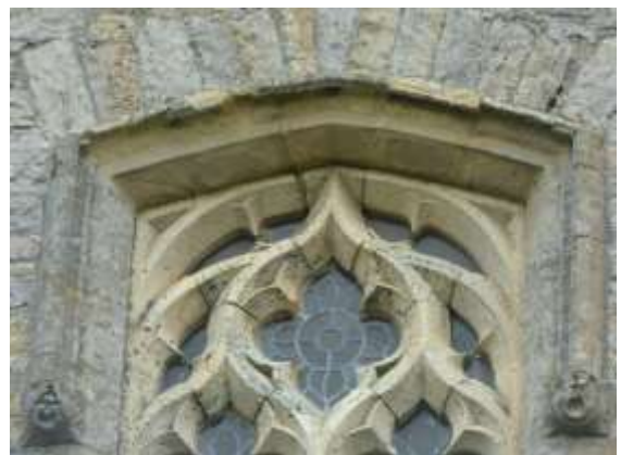
11. Close views of decayed stonework to base of spire and window.
