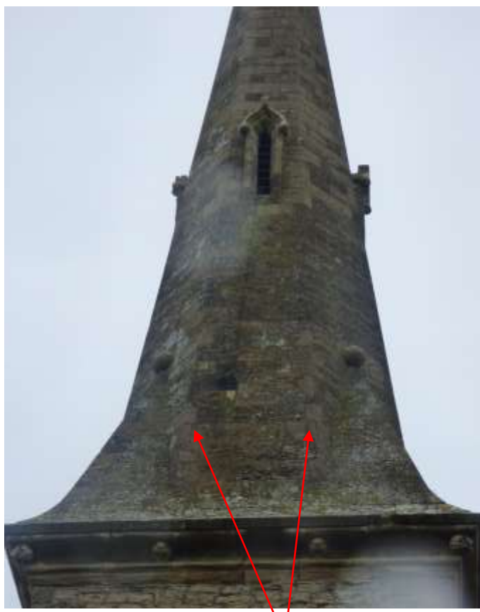
12. Further evidence of past cement patch repairs to base of east side of spire.
