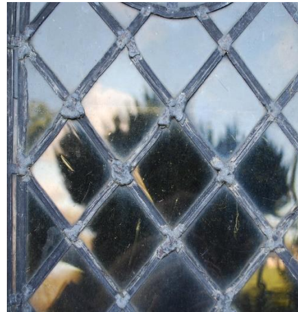
Detail from exterior, unsightly solder joints
