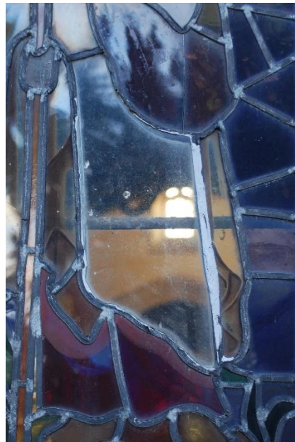
Detail from exterior, previous repair
