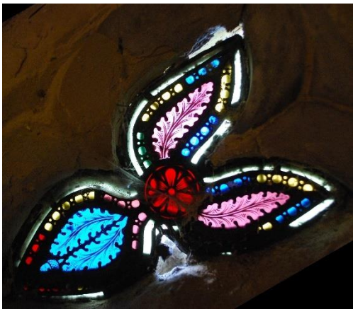
Detail, light gaps due to stonework erosion and mortar loss
