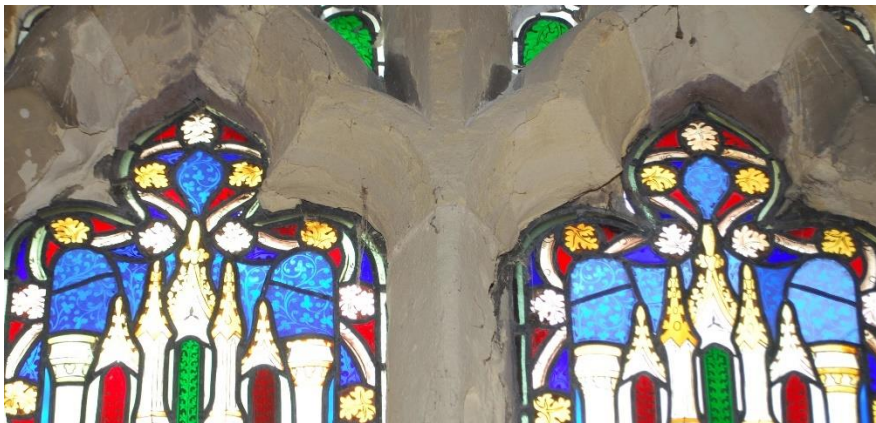
Detail, heads of lights where stonework is damaged and mortar lost
