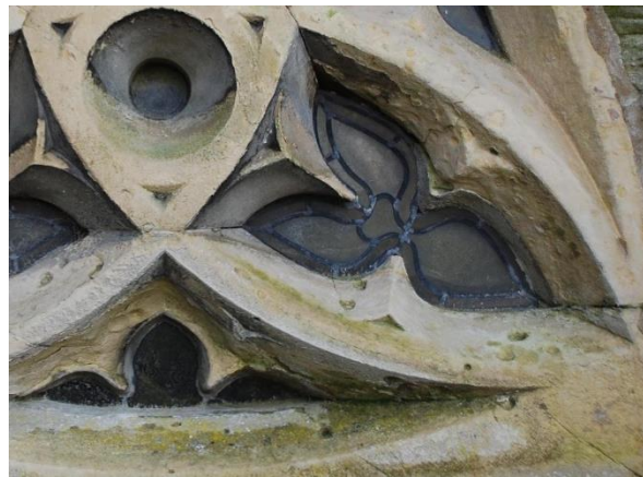
Detail from exterior, stonework erosion and algae growth due to damp conditions
